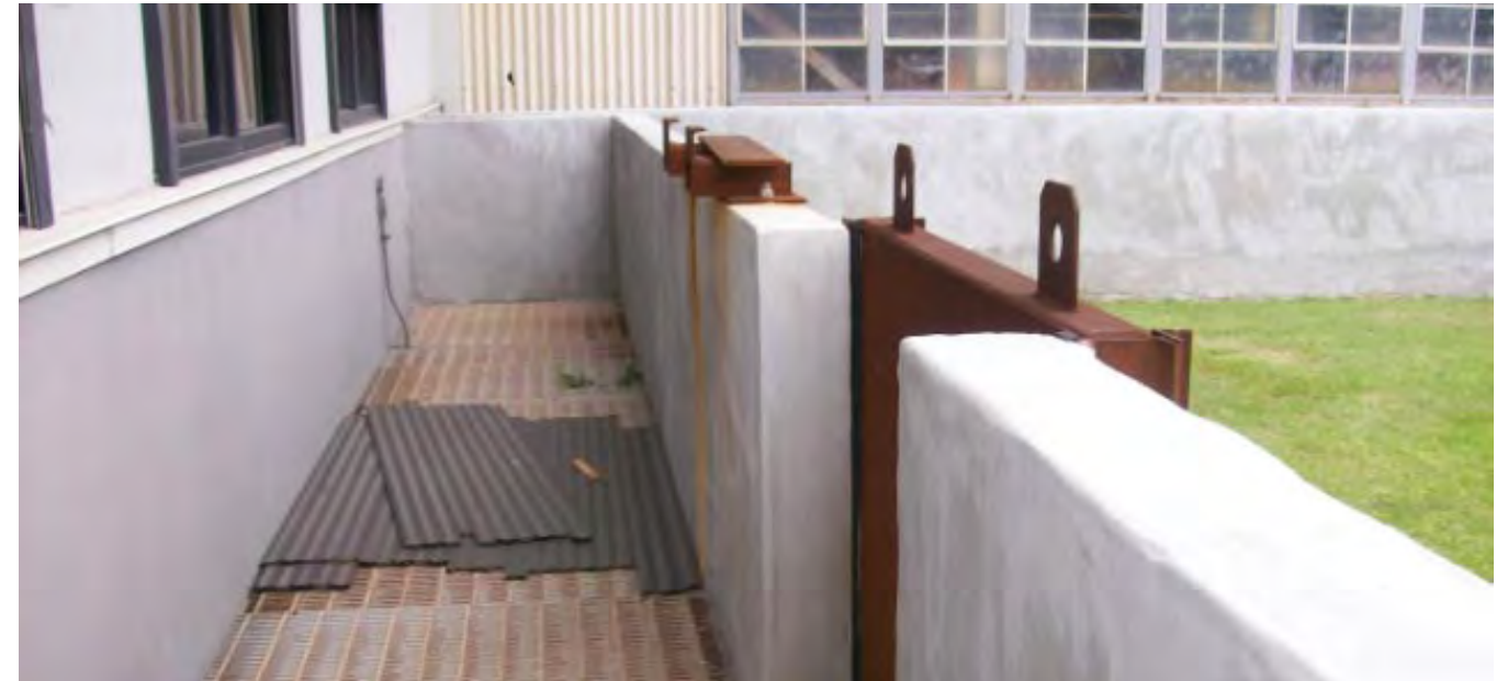
Figure 2-9 Floodproofing Wall & Gates – Slidell Memorial Hospital (NSI 2007)
